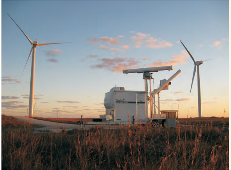
TOP: MERLIN SCADA installation at the Iberdrola Penãscal wind farm in Texas, USA.
