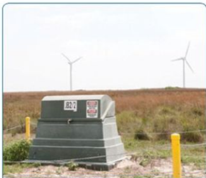
Power generated by the 118 turbines runs through 115 junction boxes to 14 different collection circuits.
