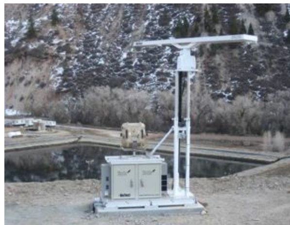
MERLIN SS200 detect & deter skid unit at Encana Middle Fork plant, Parachute, CO, USA.
