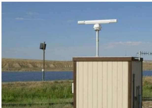
MERLIN X10 detect & deter Bird Control Radar system, PacifiCorp Jim Bridger, Cheyenne, WY USA.
