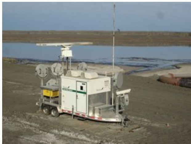
The MERLIN detect & deter Bird Control Radar system at the CNRL Horizon Mine oil tar sands facility was the first large-scale, wide area, automated bird control radar system installation in the world and has proven very effective in reducing bird mortality.
