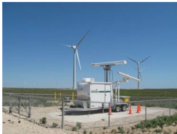
MERLIN bird radar system with MERLIN SCADA integrated with wind farm control system to automatically idle turbines when birds are detected approaching the wind farm under high mortality risk conditions.
