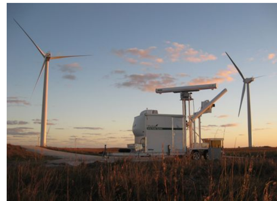
The first MERLIN SCADA radar-based mitigation installation at a windfarm in Texas, USA (2009).
